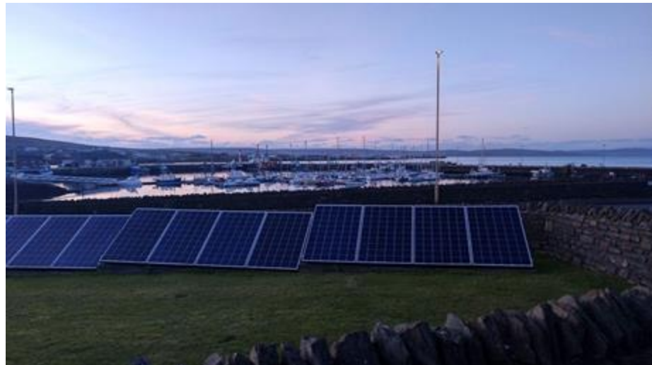
Kirkwall, Orkney, Solar panels
